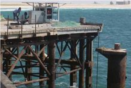
Desalting system on the harbour
