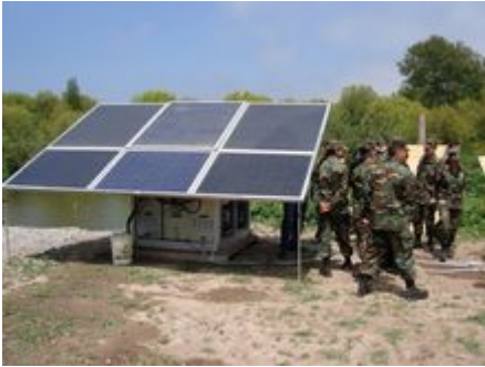
Presentation of our water desalination plant which is installed on the ground of the Chilean military training centre near by Santiago.
