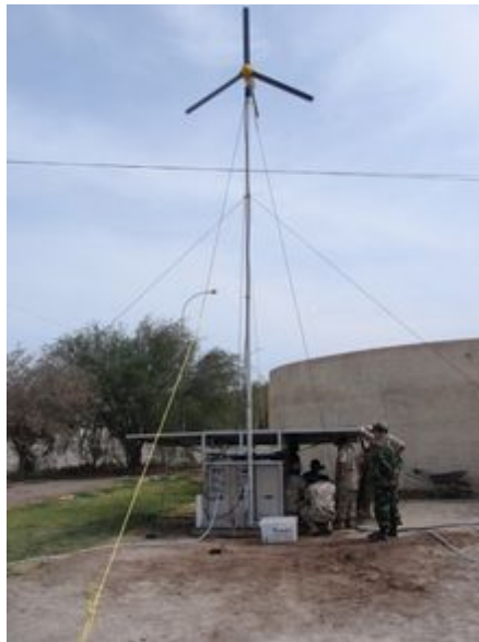
A wind generator supplies additional power up to 1000 watt per hour.
