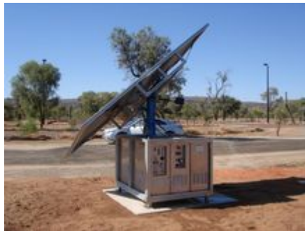
The unit treats brackish borehole water to drinking quality
