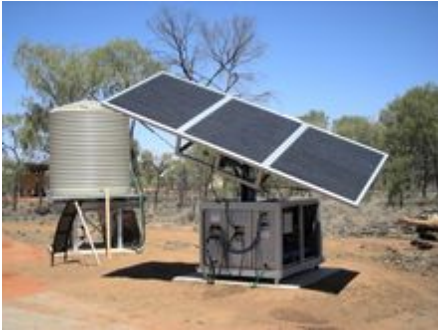
A solar powered brackish water system provides drinking water for visitors.
