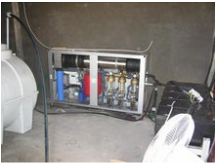
The Tank and the water treatment unit are installed at the bottom of the tower. The pump lifts the treated water up to the tank above, which has a size of 25'000 liter.
